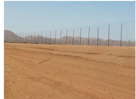
Site sub-grade had to be wet and rolled daily due to hot, dry and windy conditions
