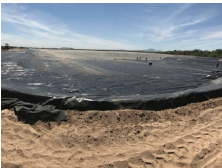
Anchor trench of pond lined with Dura-Skrim® RPP liner to prepare for anchoring the perimeter
