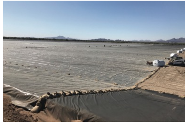
Ballast placed immediately after panel deployment due to strong winds and Dura-Skrim® RPP panels staged
